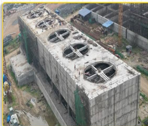
CGP Cooling Tower (CT) - B
