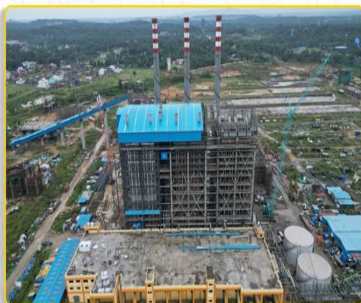
Steam Generation Plant
